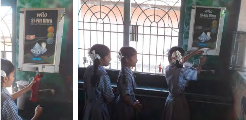
Children using water filters installed under URMEE project
